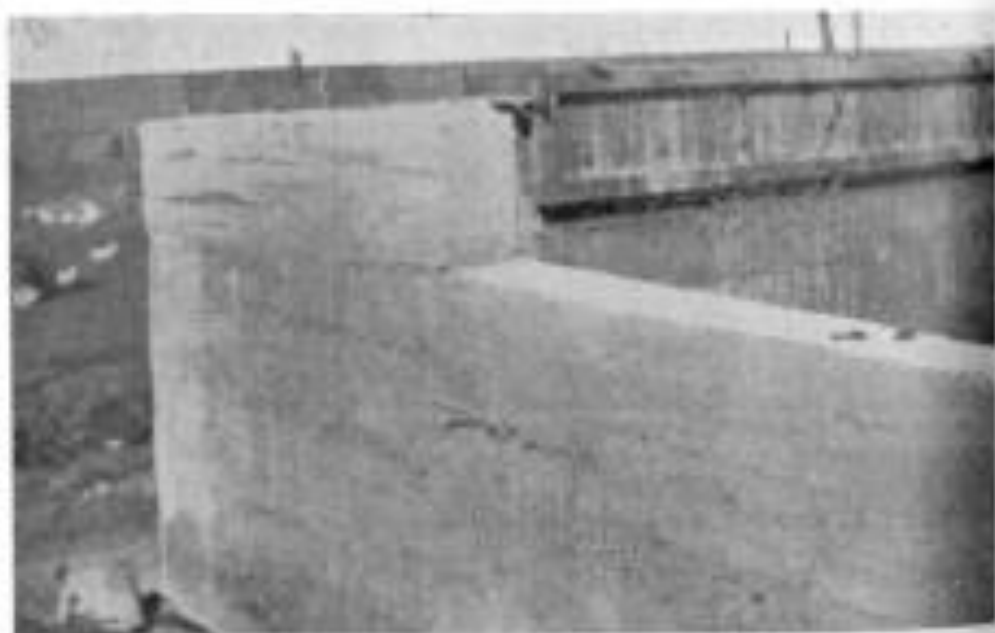
Fig. 2.—The moulds must be square at the corners. Note the appearance after removal of the mould at the corner.
